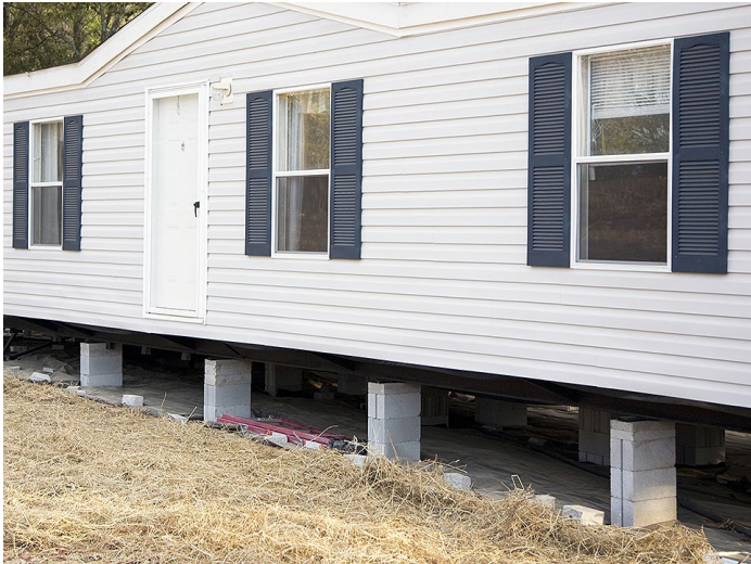
Up on blocks, but not on concrete pad
