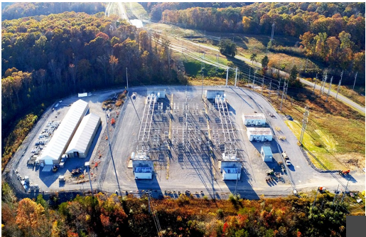
Substation sensor testing
