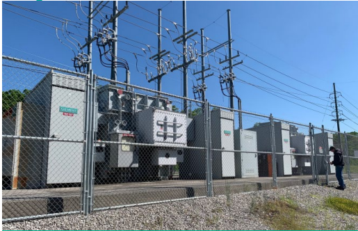
Fully instrumented substations with sensor testing
