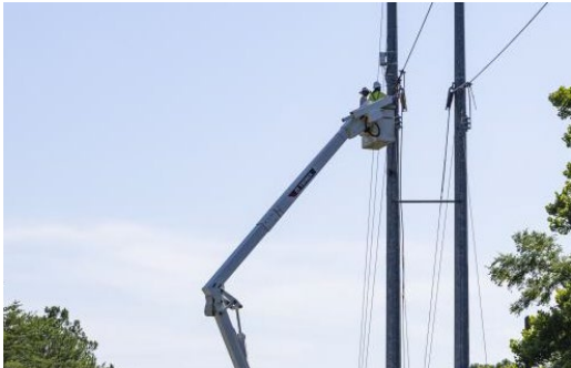
PCAT Novel conductor testing
